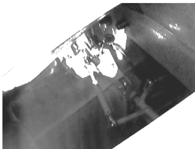
ABOVE: The mixer section and an indication of the size of the access hatch area for working inside this area.
