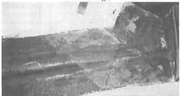
Photo 3 - Second layer of fiberglass cloth laid on at a 45° angle the other way.
