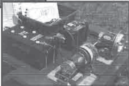
Close up of the system with the big, Super Crank 1,300 amp marine-commercial heavy duty battery.
